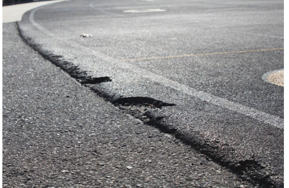
The school track with rough and crumbling edges. It is planned to be resurfaced in 2028. Photo by Aspen DeWan.
