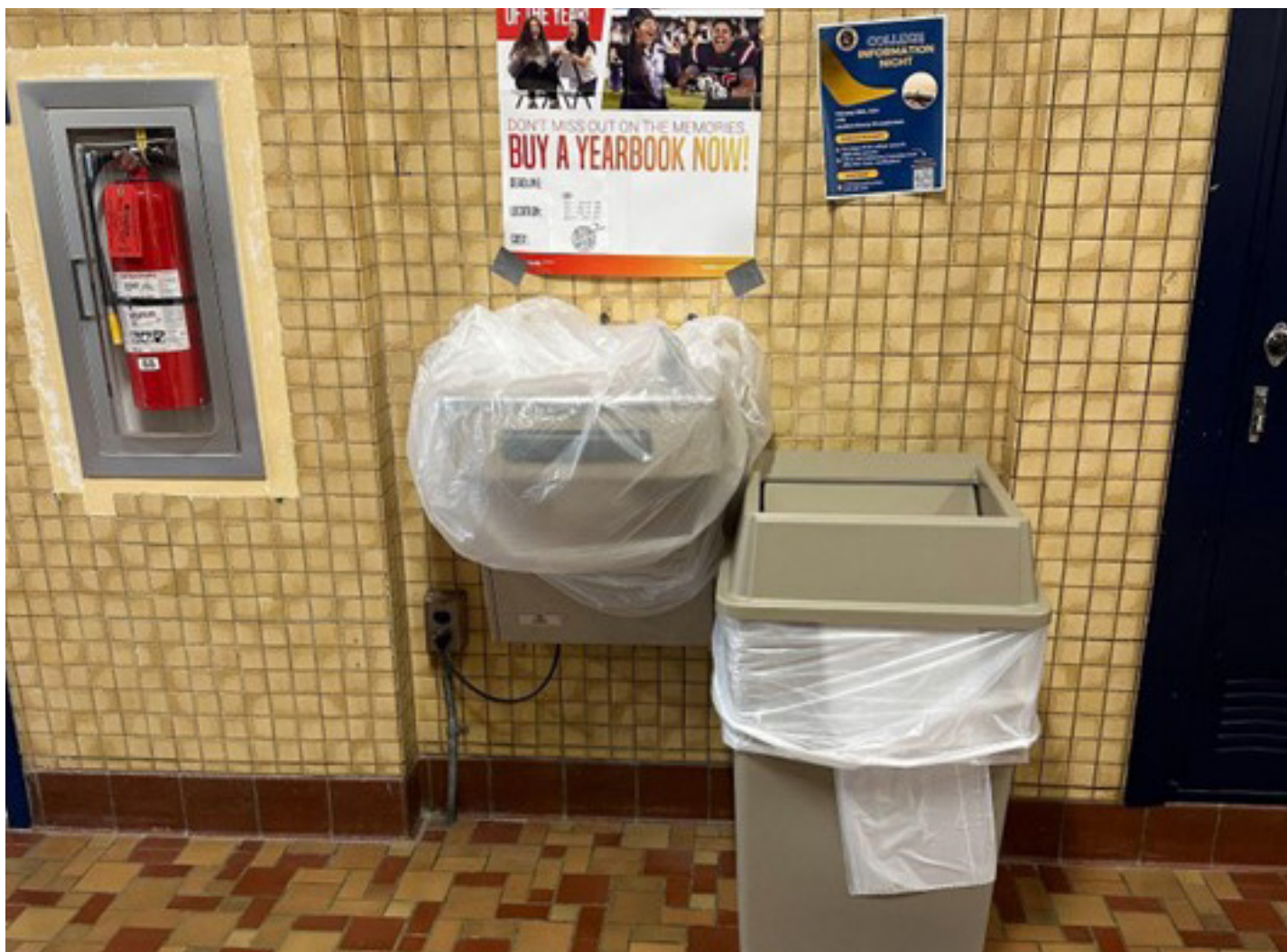
A water fountain on the second floor is closed off, as the water is not currently safe for drinking. After a recent illness that spread, swiftly, throughout the entire school, health specialists have taken the matter into their own hands, and are currently investigating the cause of this virus. Photo by Karan Singh.
